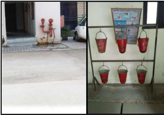
Fire Fighting Equipment
